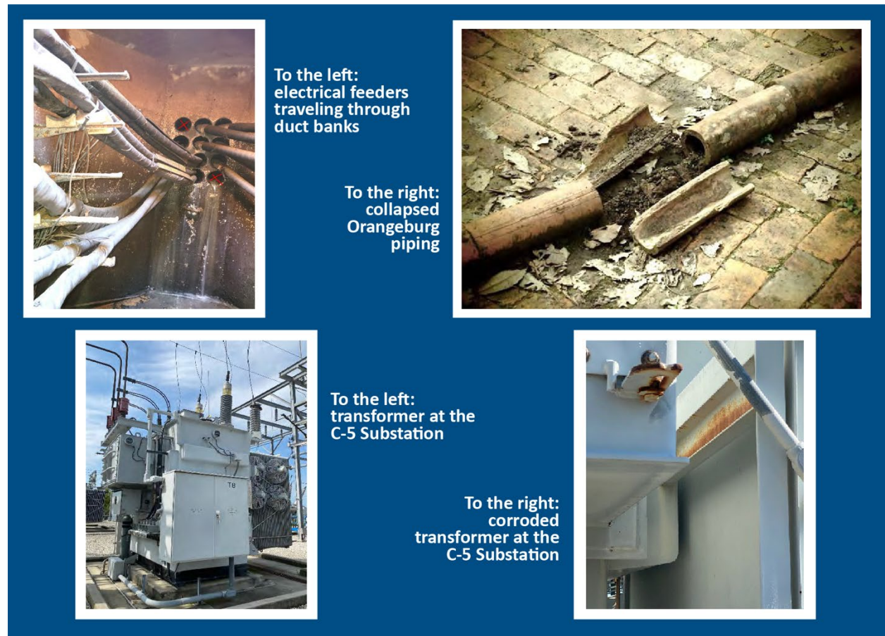
Figure 7: Examples of Collapsed Duct Banks and Corroding Transformers at Kennedy
