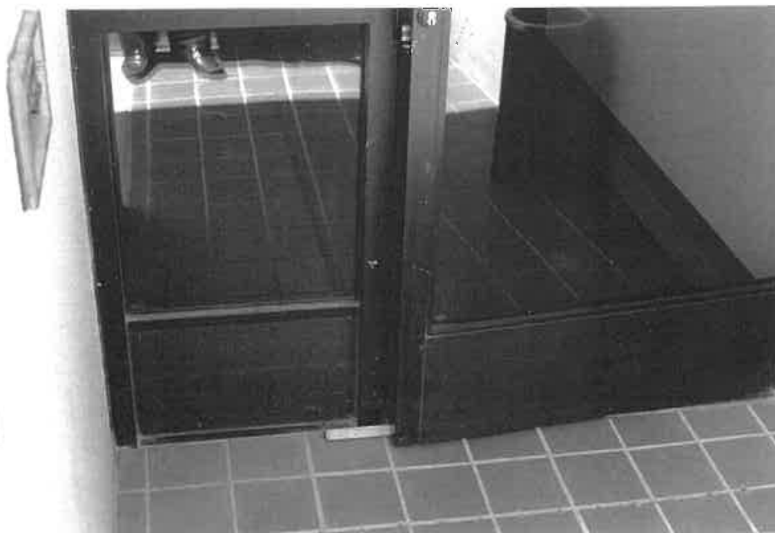
PIECE OF WOOD IN DOOR AT NAS SUPPORT BUILDING A
