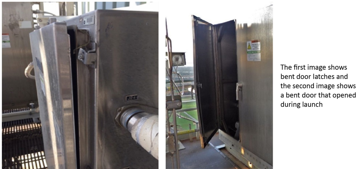
Figure 6: ML-1 Panel Door Damage Post-Artemis I Launch
