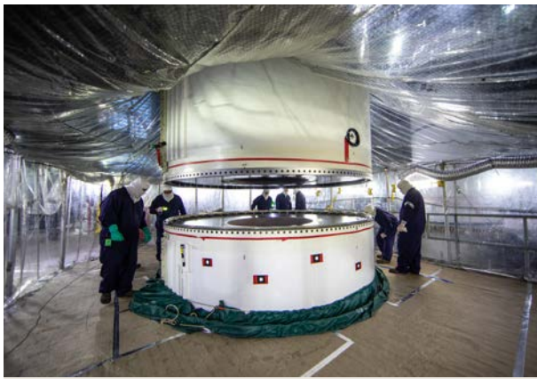
Workers with Exploration Ground Systems and contractor Jacobs teams assist as the right-hand forward segment for NASA’s Space Launch System is lowered onto the center forward segment on the mobile launcher at NASA’s Kennedy Space Center on February 23, 2021.
