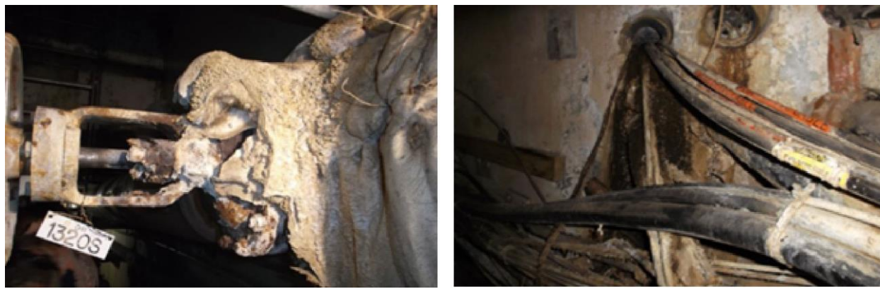
Figure 2: High Pressure Lines in a Langley Research Center Utility Corridor
