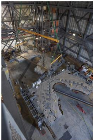
Work platforms inside the VAB provide access to the Space Launch System core stage and solid rocket boosters during processing and stacking operations.
