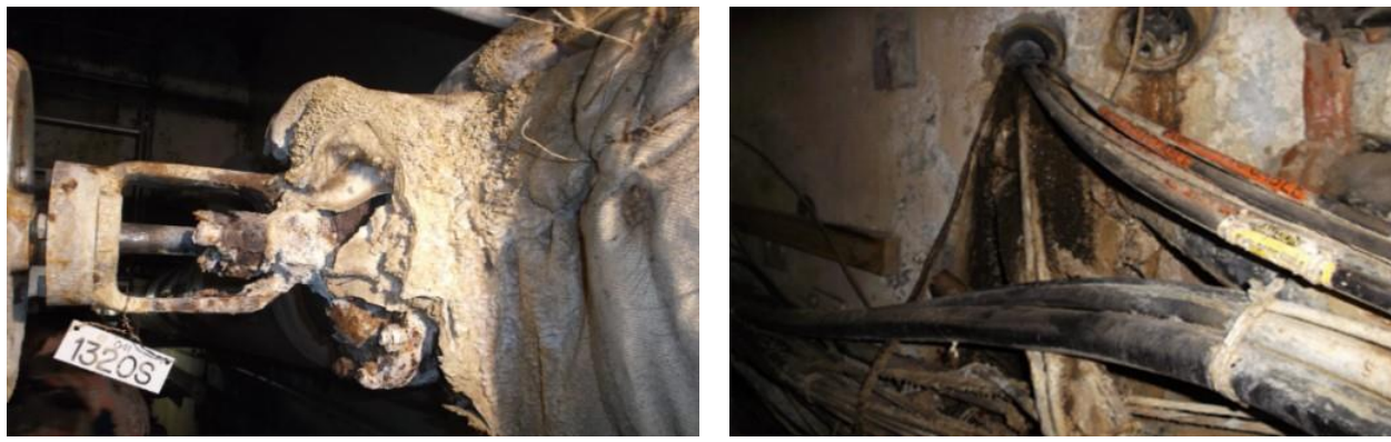
Figure 4: High Pressure Lines in a Langley Utility Corridor
