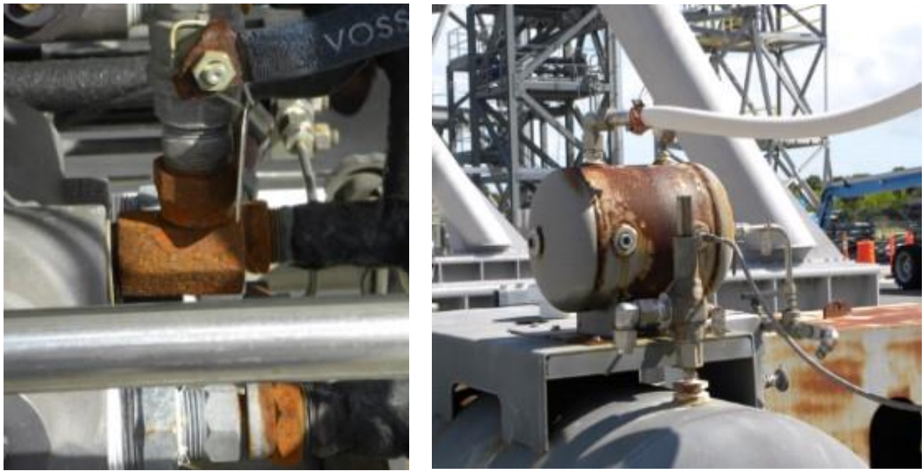
Figure 6: Corroded PVS Components at Kennedy
