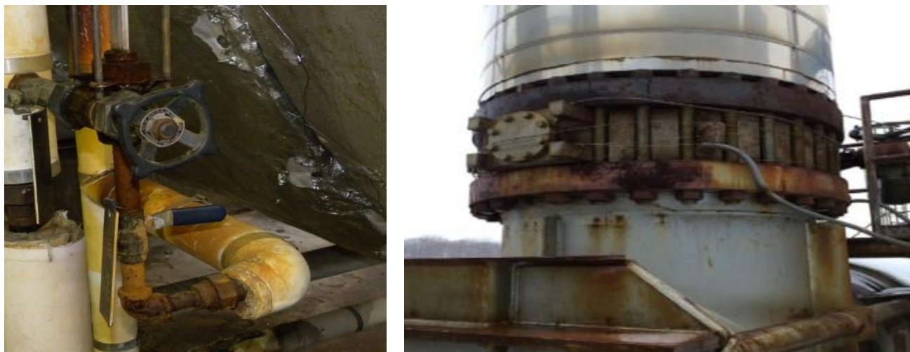
Figure 7: Corroded PVS Components at Glenn
